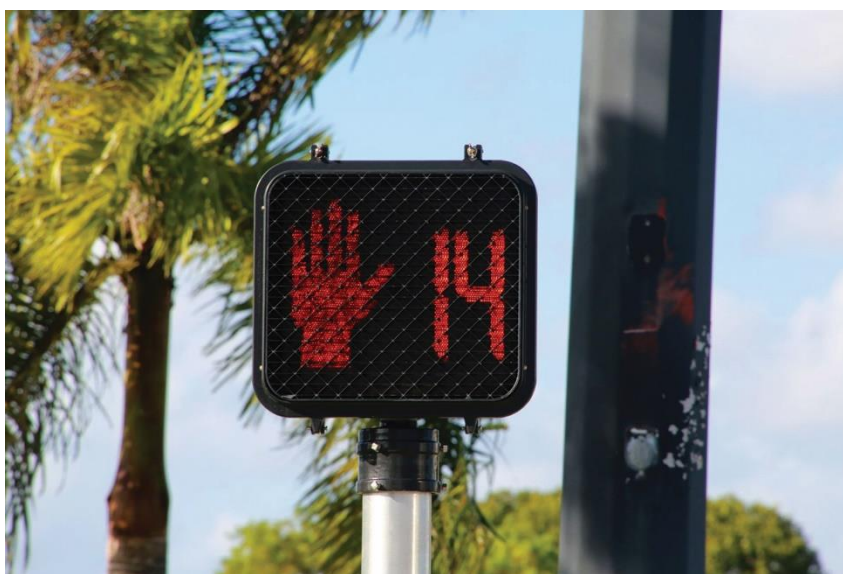
Figure 28: Example of Pedestrian Countdown Signal Head at an Intersection
