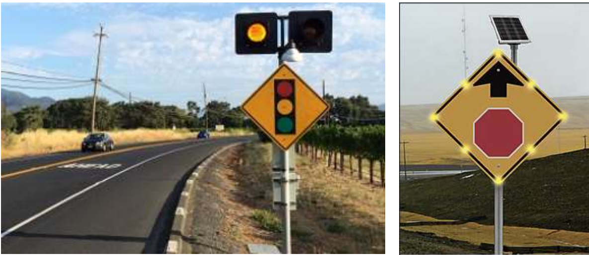
Figure 19: Example of Flashing Beacons or LED Lights as Advance Warning to Intersection
